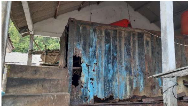
Figure 11. Broken ice factory
